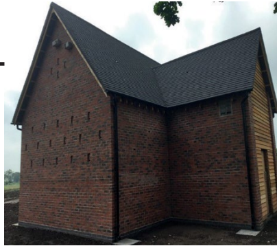
Drayton Basset - Completed Bat Barn CLM poured the first concrete for HS2 on the Enabling Works North for LMJV during the construction of Drayton Basset Bat Barn.
