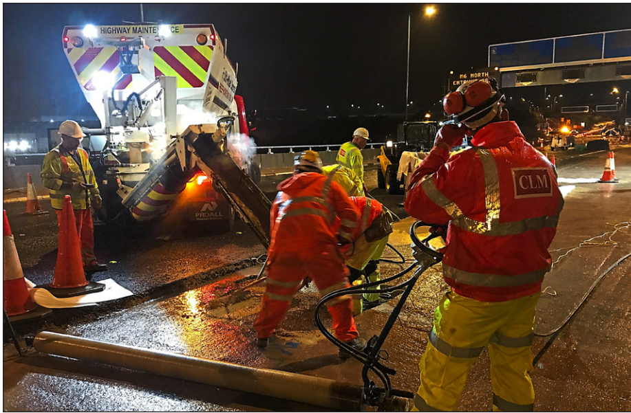
CLM's innovatory use of a rapid setting concrete significantly reduced delays to the public on Birmingham's key arterial route to the M6
