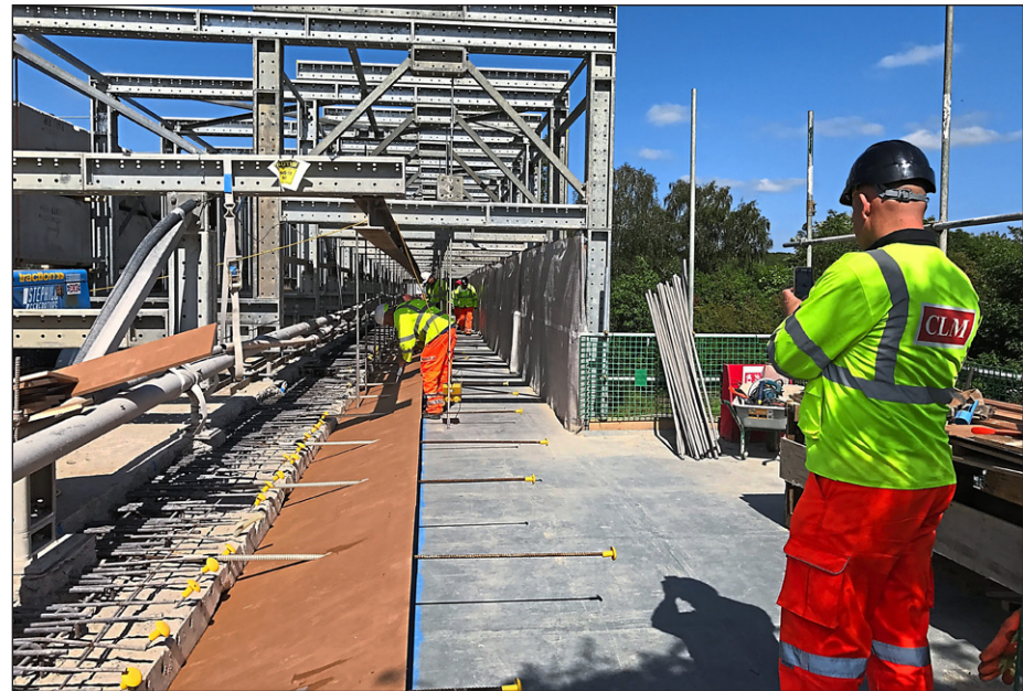
CLM replacing sections of M50 over bridges whilst keeping the traffic moving below
